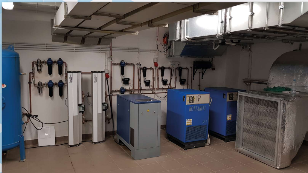
Medical air plant
