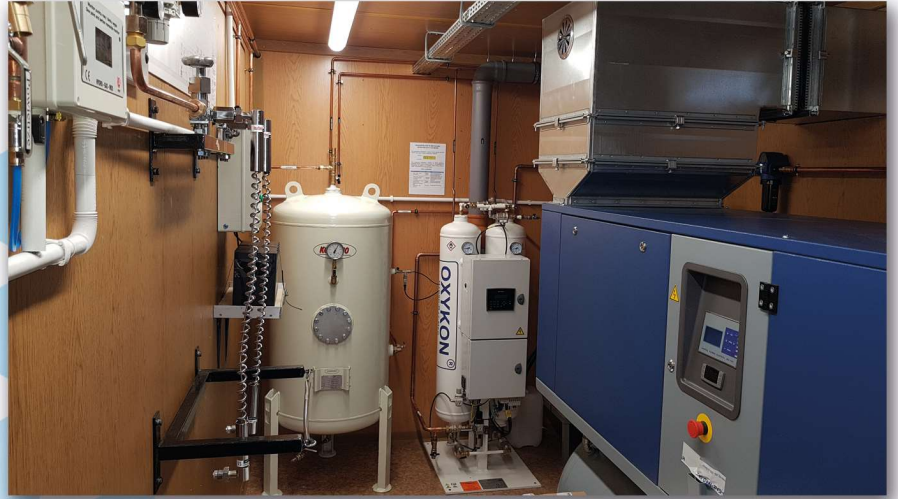
Oxygen concentrator system in container
