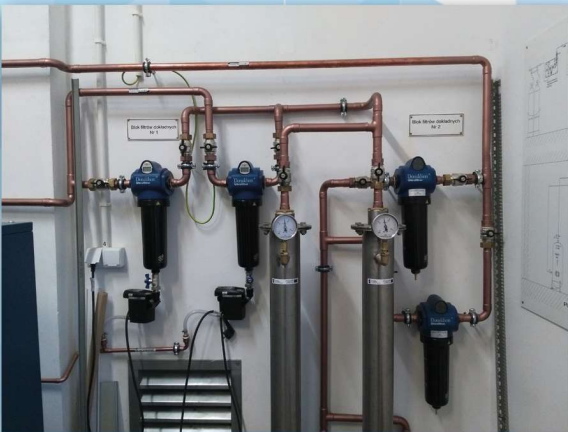
Compressed air treatment
