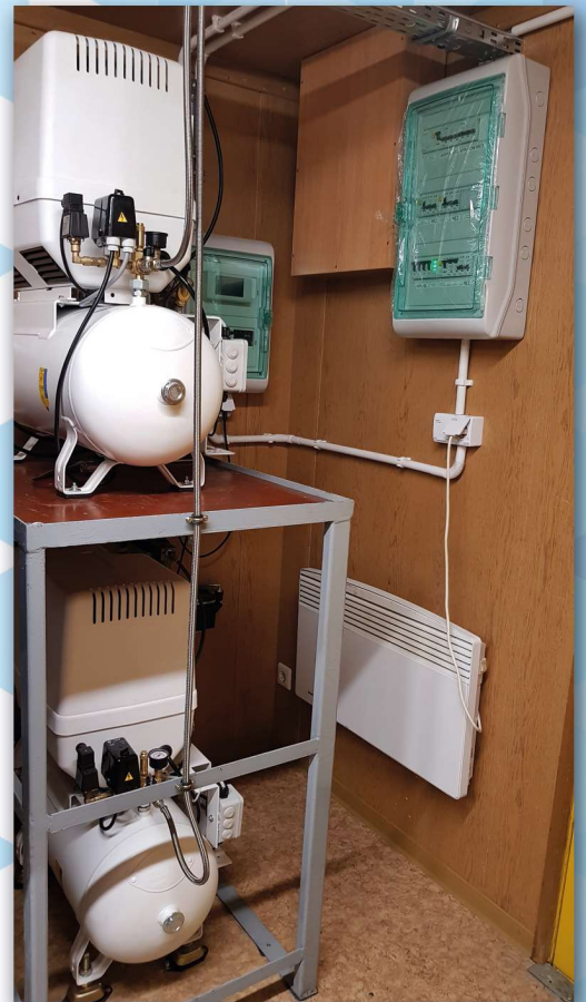
Medical air system in container
