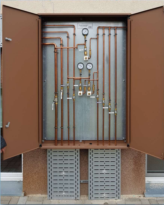
Maintenance and emergency node
