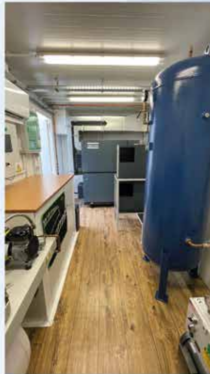
Compressed air system
