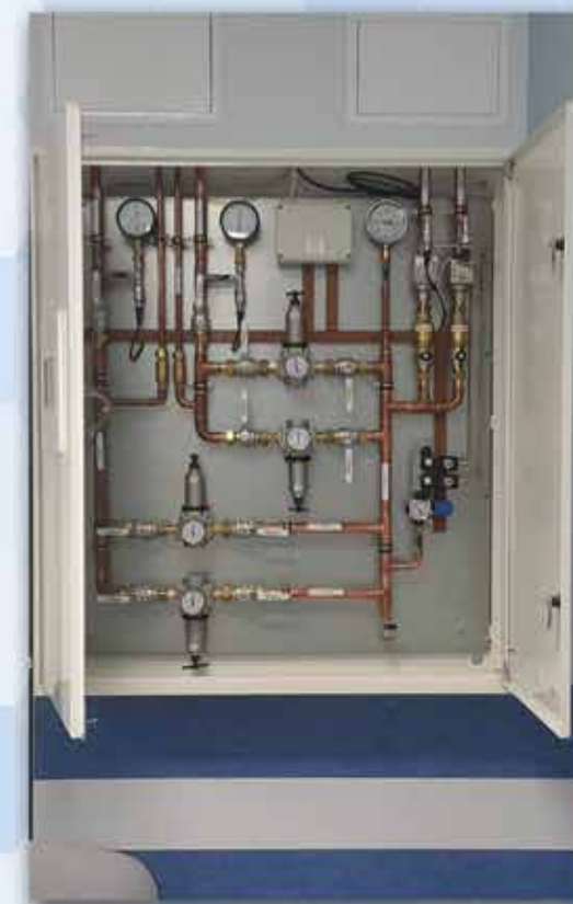
Oxygen control panel
