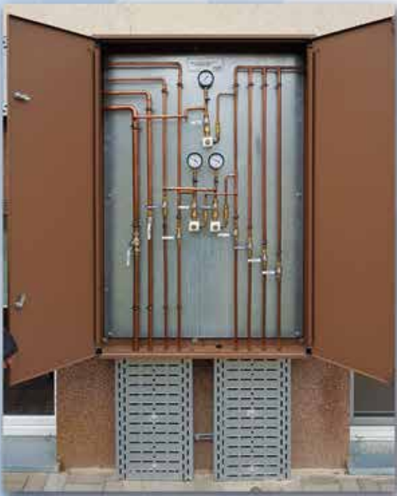
Maintenance and emergency node
