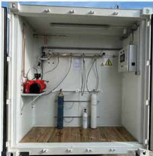
Cylinder filling station
