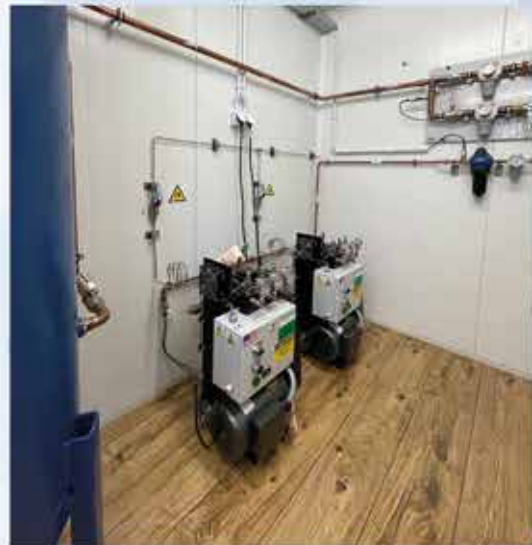
High pressure compressors
