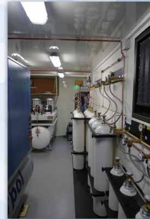
Oxygen concentrator and cylinder filling system in container
