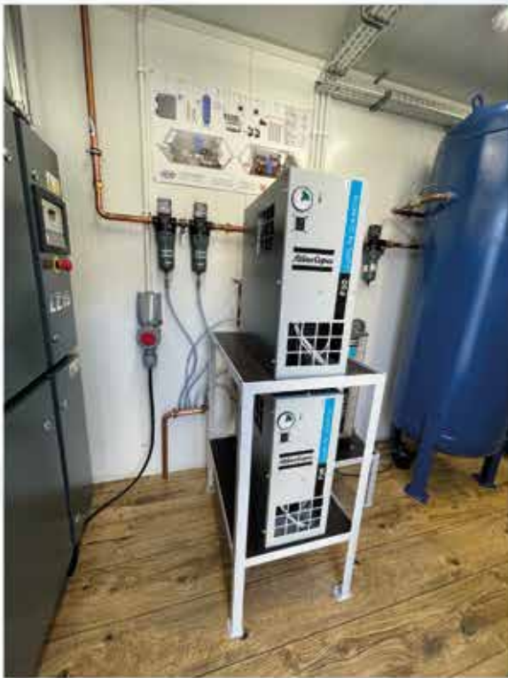
Compressed air system
