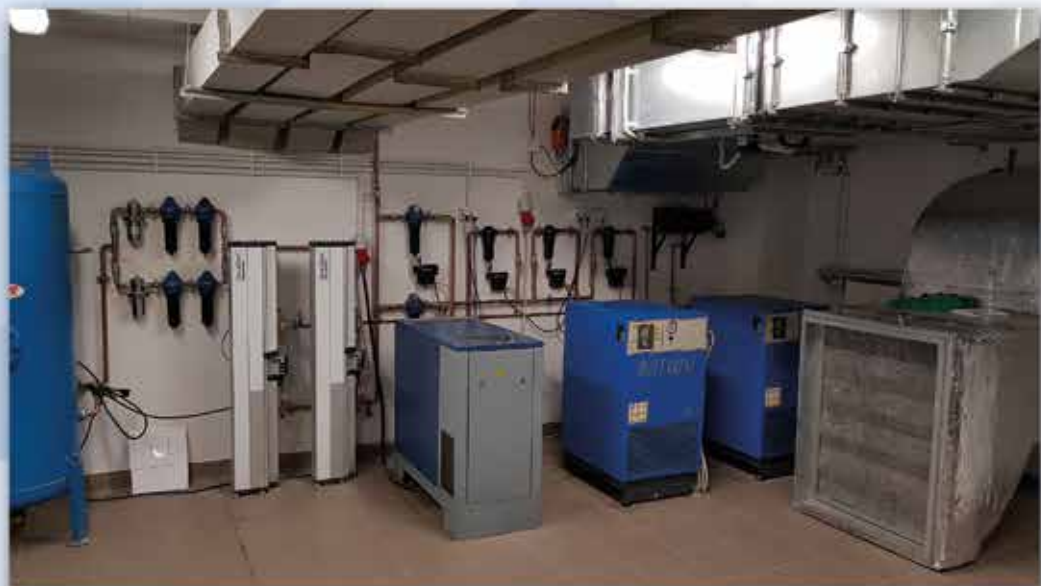
Medical air plant
