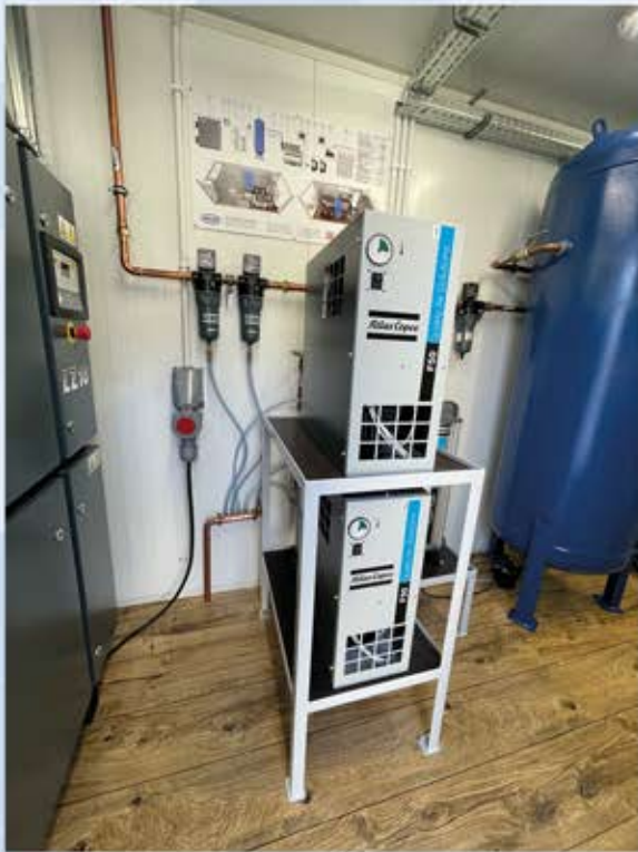
Compressed air system
