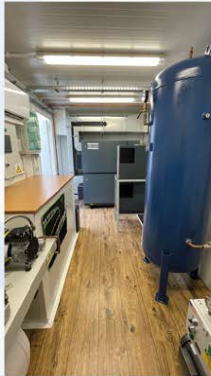
Compressed air system
