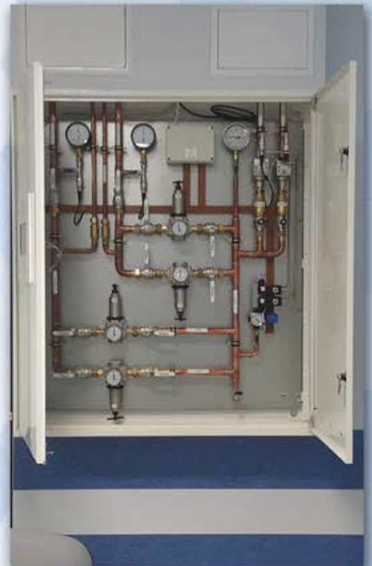
Oxygen control panel
