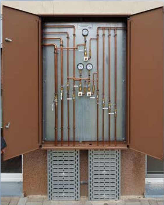
Maintenance and emergency node
