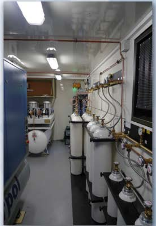
Oxygen concentrator and cylinder filling system in container
