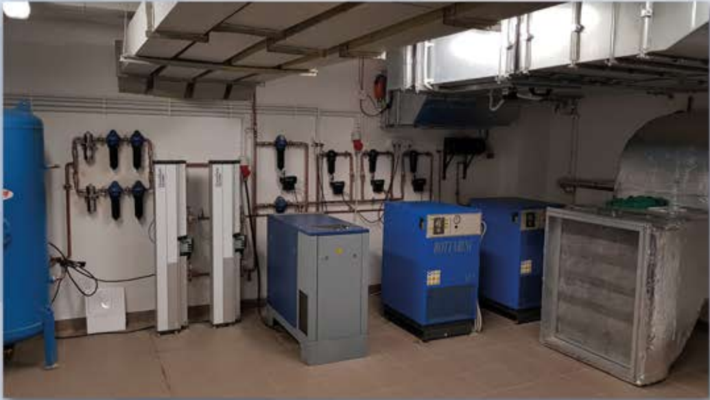
Medical air plant
